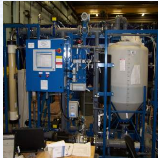
Combined Primary & Secondary Concentration on a single skid Field Evaluation ASCF 1 – 2.5 m 3 /hr
