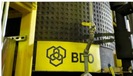
Integrated Demo Plant – 2011
